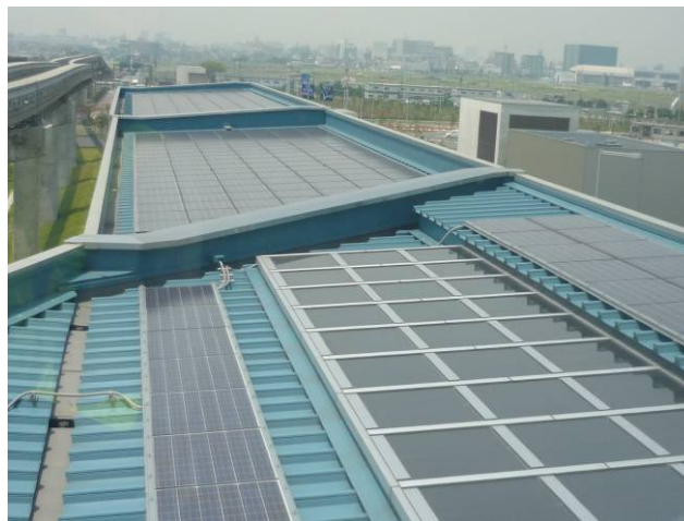
Solar power generation facilities
